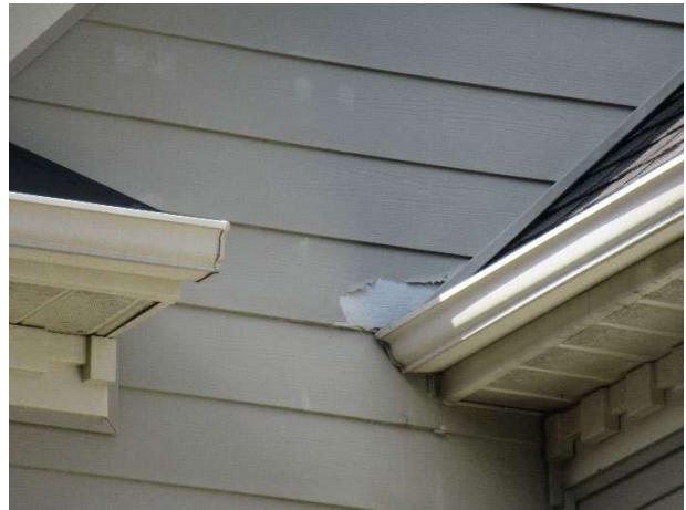
Peeling paint finishes
