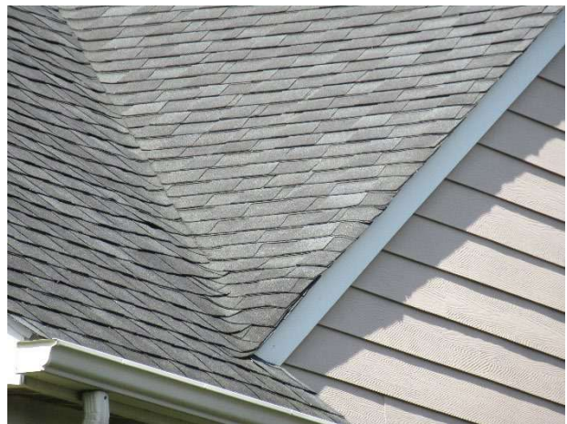
Curled shingles at single family home
