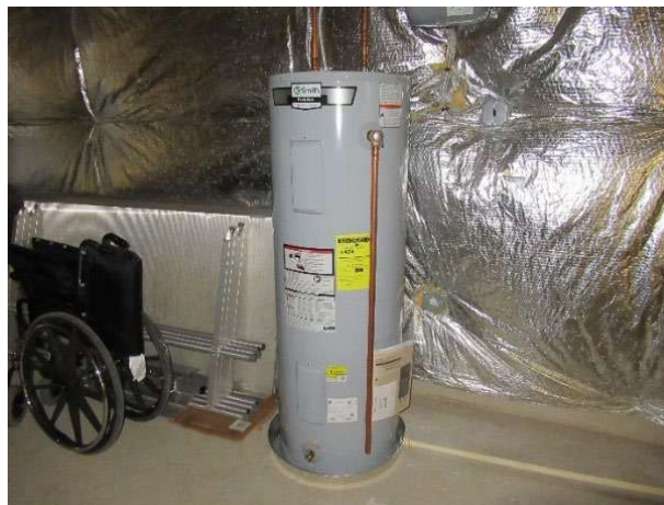
Water heater overview
