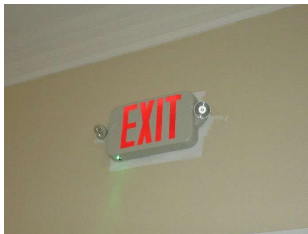
Exit and emergency light fixture
