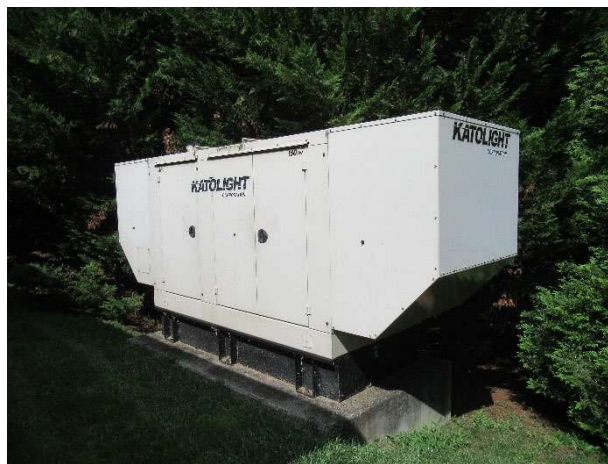
Emergency generator overview
