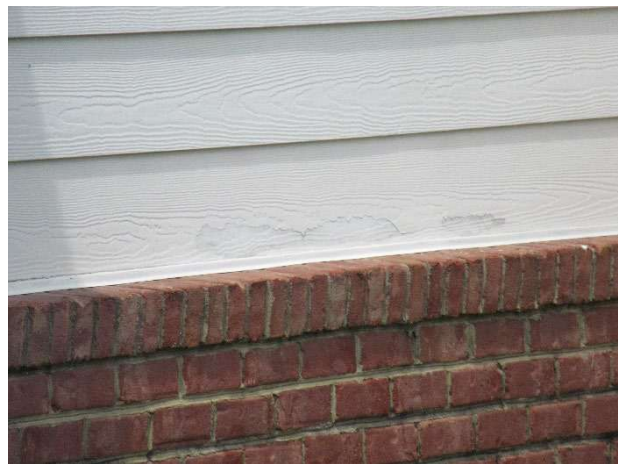
Peeling paint finishes
