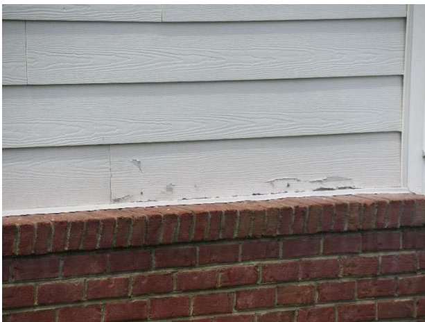
Peeling paint finishes
