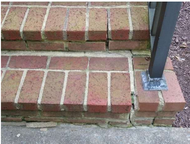
Mortar deterioration and displaced bricks
