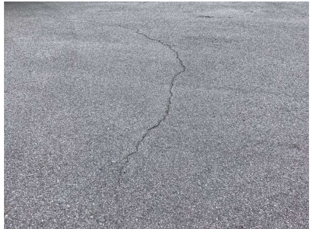
Pavement cracks at street
