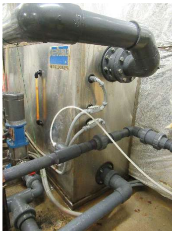
Air stripper aeration tank
