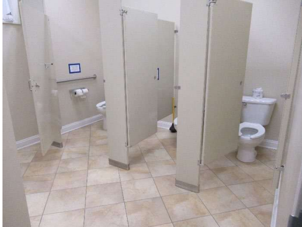
Rest room fixtures and partitions
