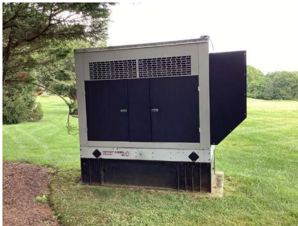
Emergency generator overview
