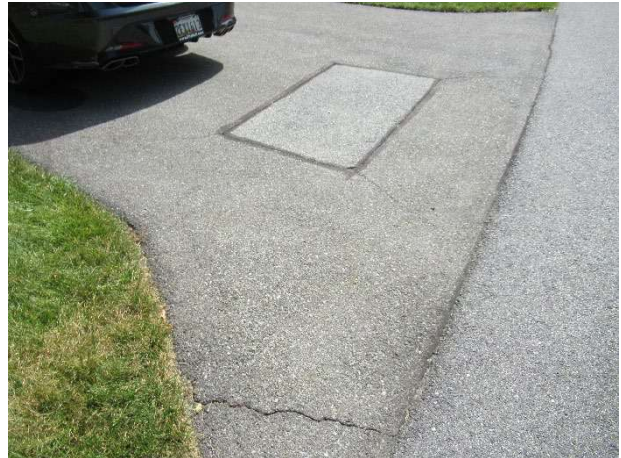
Pavement cracks and patching at driveway
