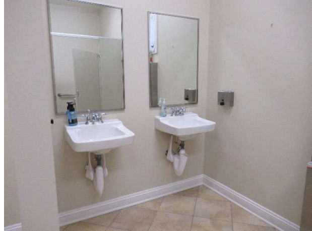
Rest room fixtures
