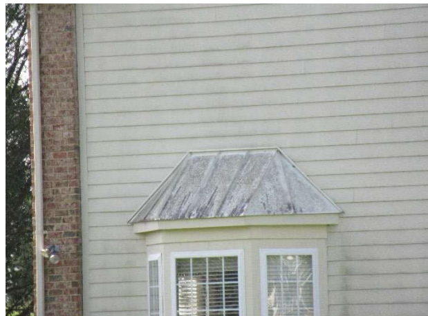
Metal roof overview – Note: finish deterioration
