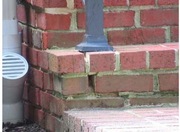
Mortar deterioration and displaced bricks
