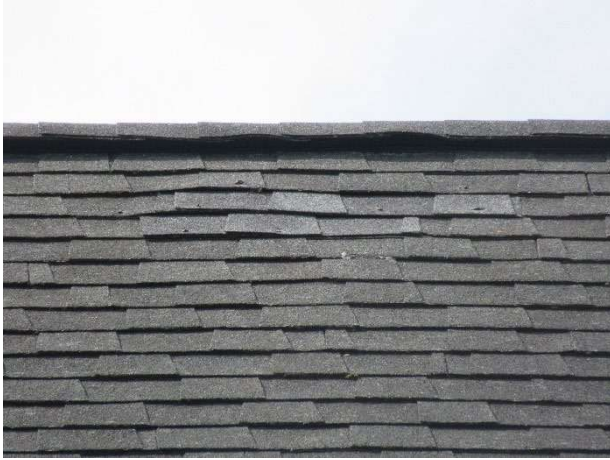
Curled shingles at townhome roof
