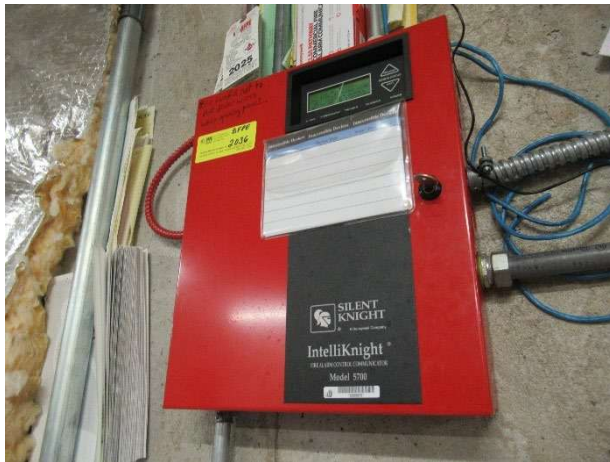
Fire alarm control panel overview
