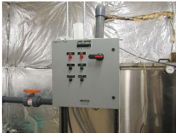
Air stripper controls
