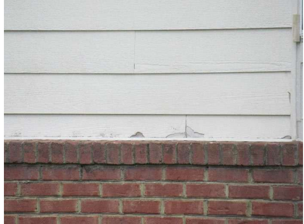
Peeling paint finishes
