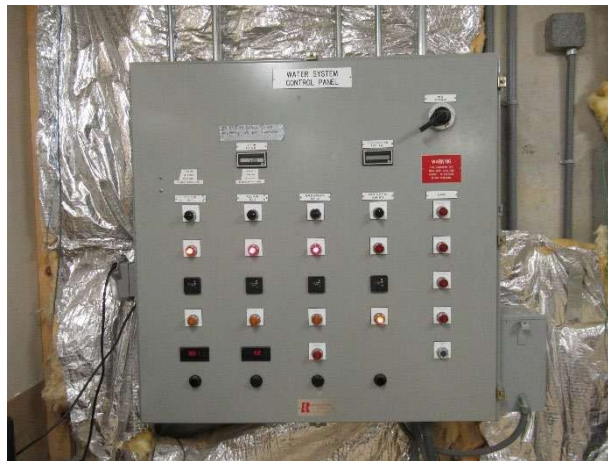
Water treatment plant controls
