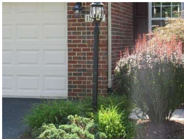
Minor light pole lean
