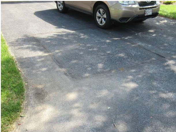
Pavement patching at driveway
