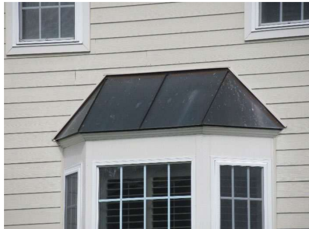
Metal roof overview – Note: finish deterioration
