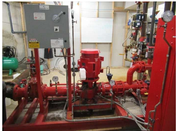
Fire suppression pump and piping
