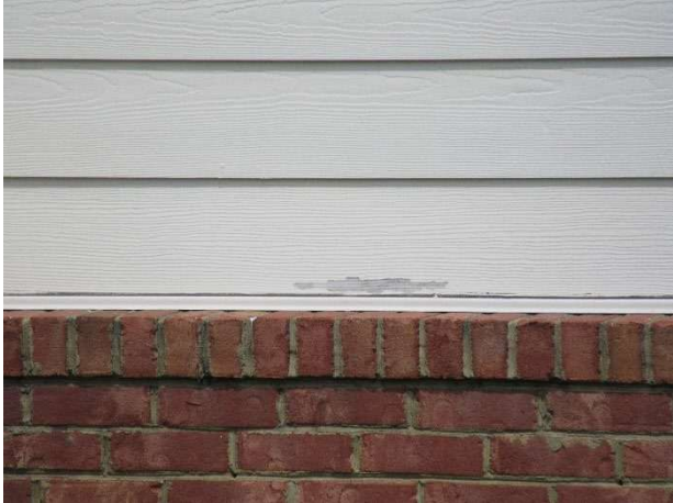
Peeling paint finishes
