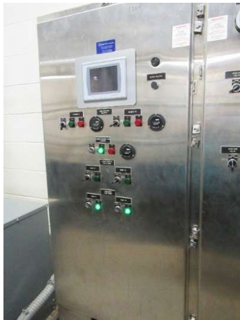
Wastewater treatment control panel
