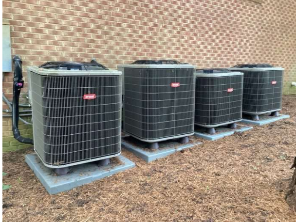
Split system condensing units
