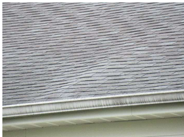
Sheathing deflection at townhome roof
