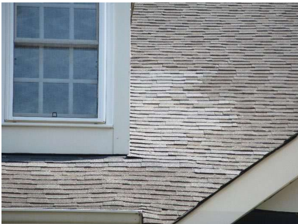
Curled shingles and partial replacements at townhome roof
