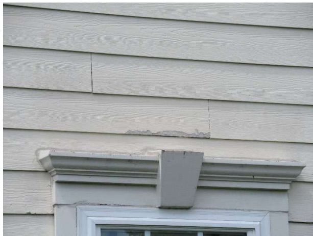
Peeling paint finishes
