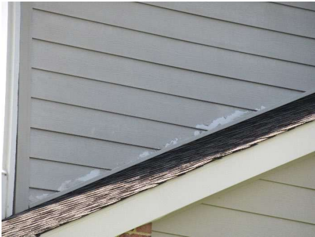
Peeling paint finishes
