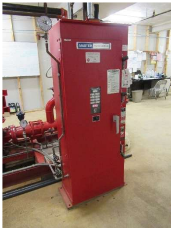
Fire suppression pump controller
