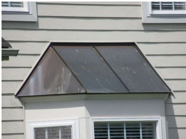
Metal roof overview – Note: finish deterioration
