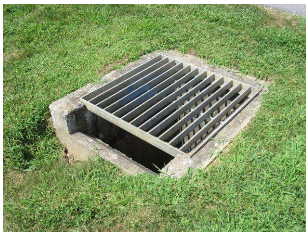
Landscape catch basin -- Note: We recommend the Association budget for inspections, repairs and regrading around these basins through the operating budget as needed.
