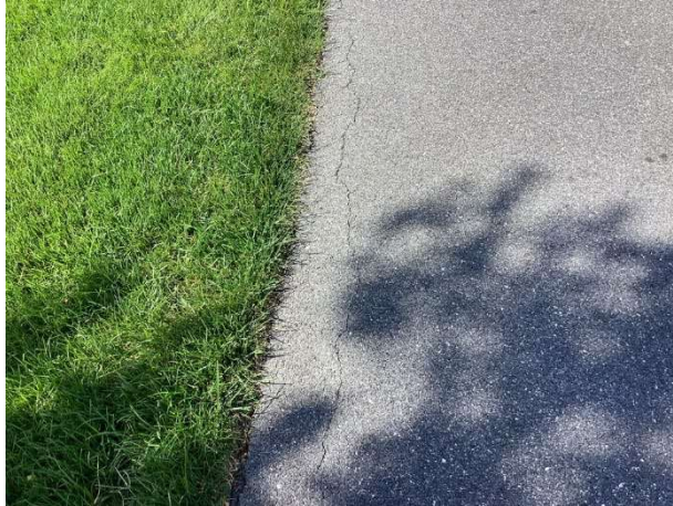
Pavement cracks at street
