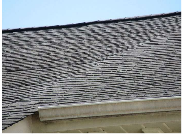
Sheathing deflection at townhome roof
