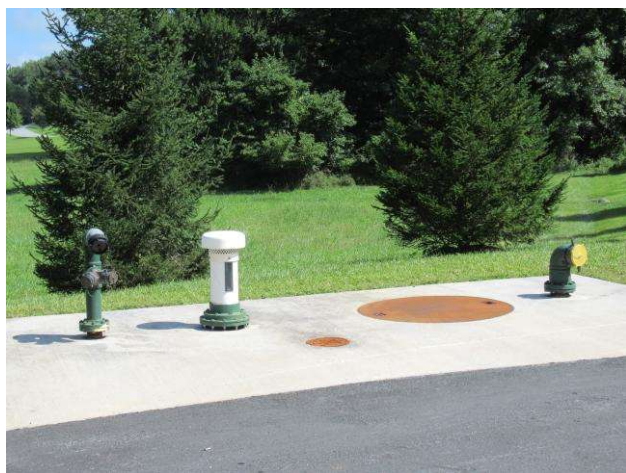
Fire department connections -- Note: We do not anticipate total replacement during the next 30 years.
