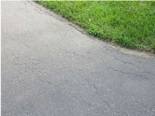
Pavement cracks at driveway
