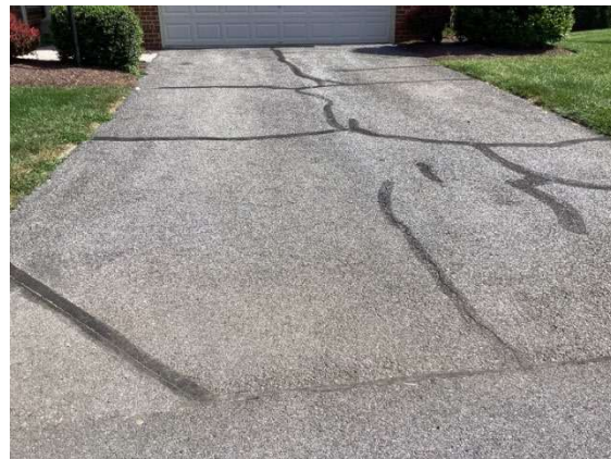
Asphalt pavement driveway overview – Note: previous repairs
