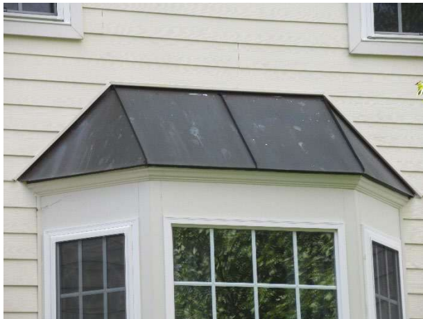
Metal roof overview – Note: finish deterioration
